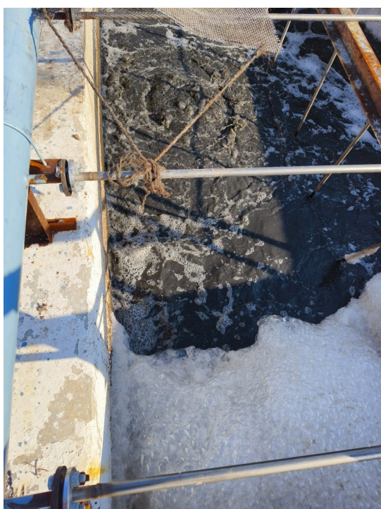
Aeration Tank - Day 1 Black inlet effluent
