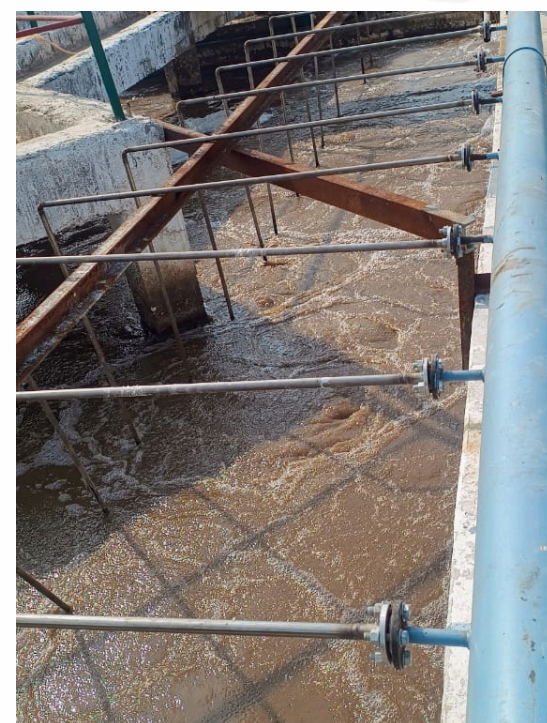
Aeration Tank - Day 7 Brown inlet effluent
