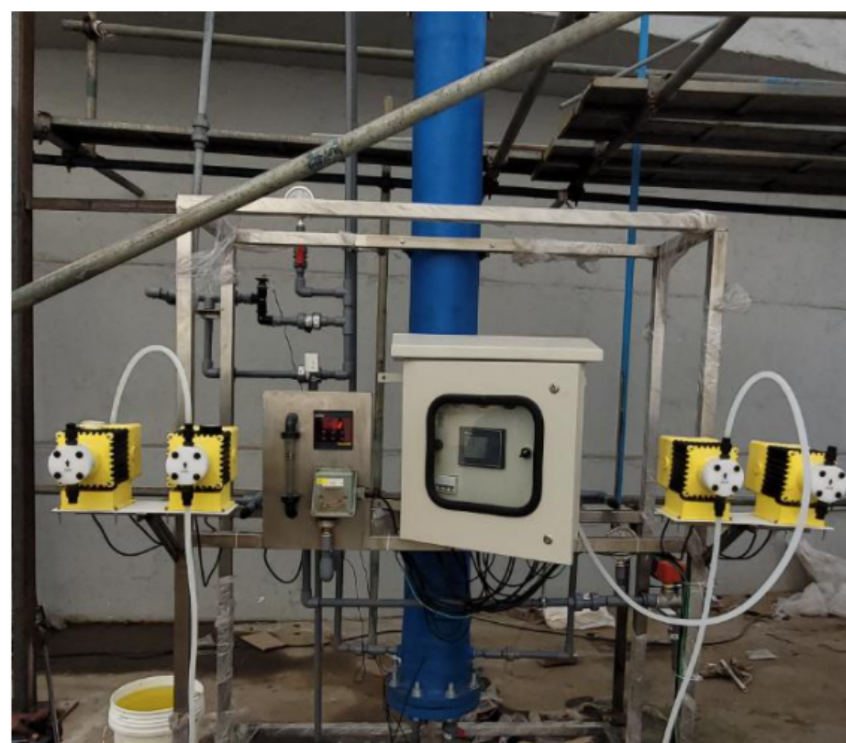
PureOx ClO 2 Generator - Installed at site
